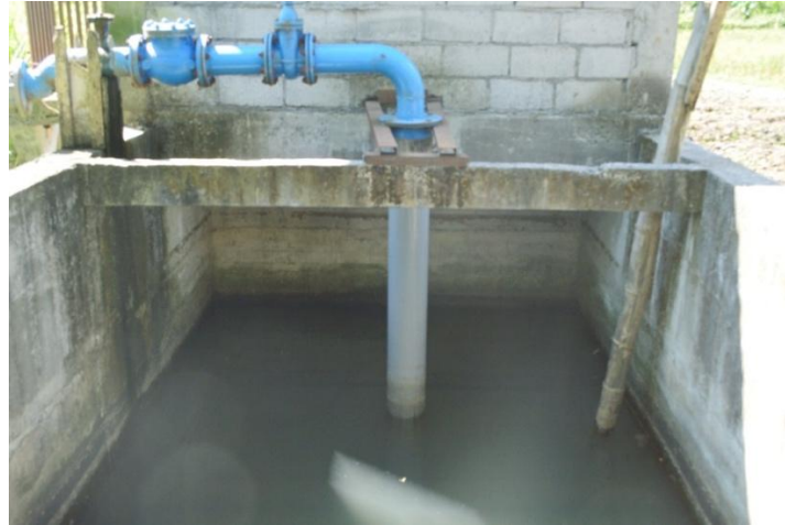
Figure 5. Photo of Irrigation Pump
